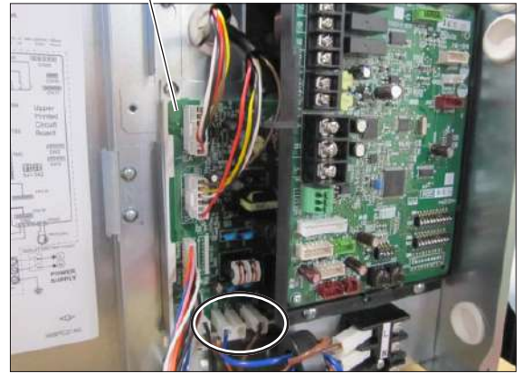
Power circuit board
