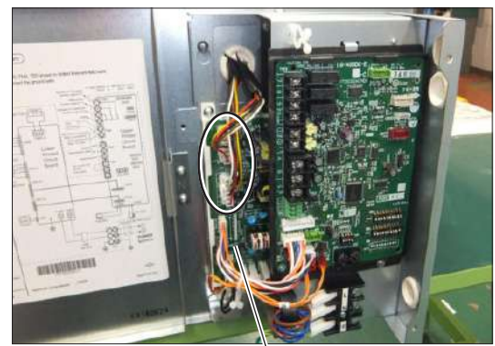
Power circuit board
